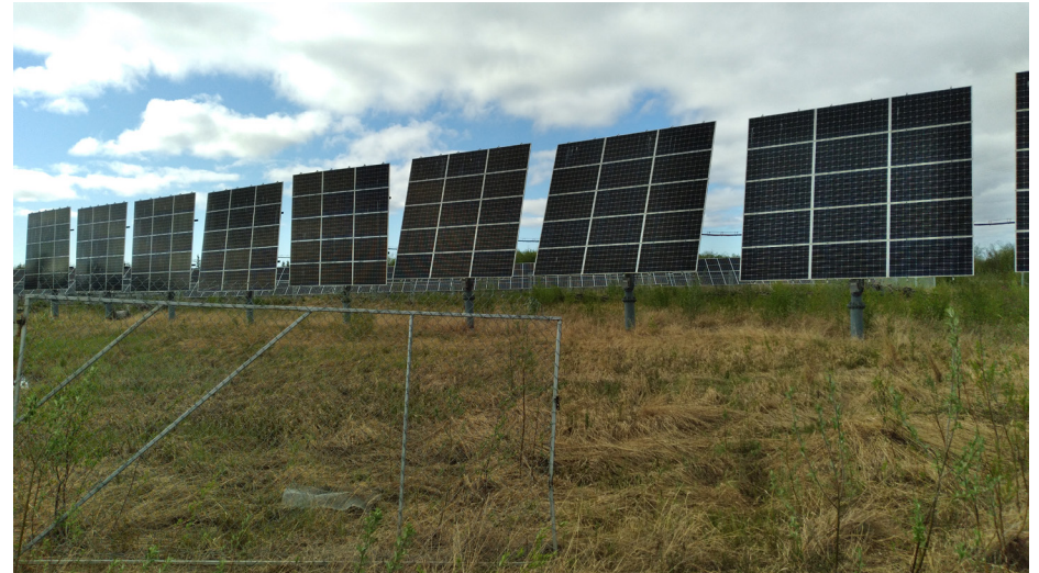
Aklavik, NWT solar project which features a 55kW ground-mounted solar array, integrated into the community's microgrid and is operated by the Northwest Territories Power Corporation.
